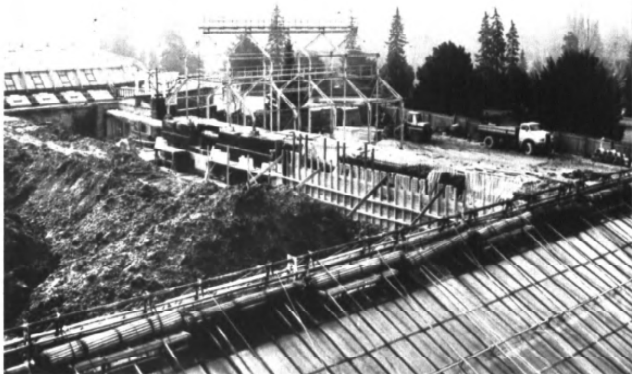
Demolition of the ancient glasshouses for Succulents. Actually these three houses are being restored.
